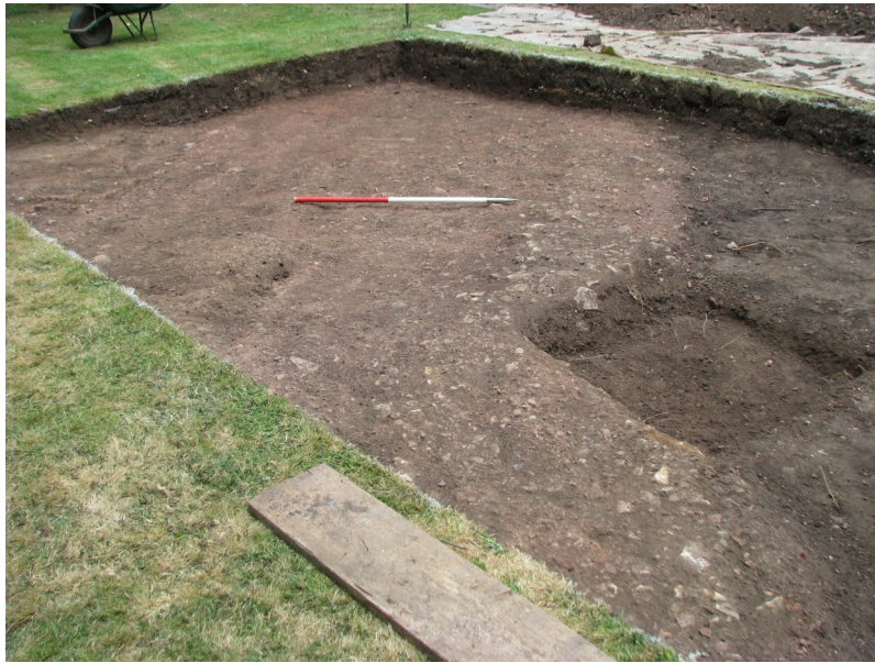
Fig 16 Topsoil removed to show the track of the contractor's road (left) and the test pit. The red-brown colour of the road is burnt shale.
