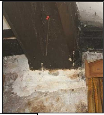
Evidence in a side wall of the ceiling level of Room 4 having been raised.
